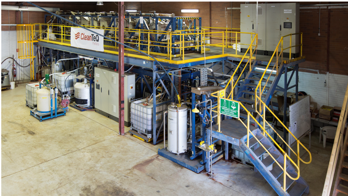
Clean TeQ's cRIP Pilot Plant in Perth, Australia
